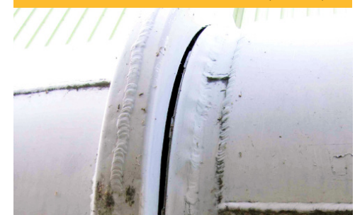
PROBLEM: CRACKED BELLOWS (METAL)
