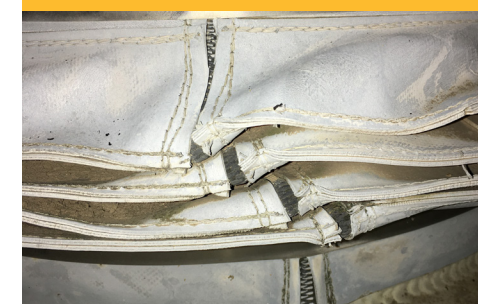
PROBLEM: DEGRADED BELLOWS
