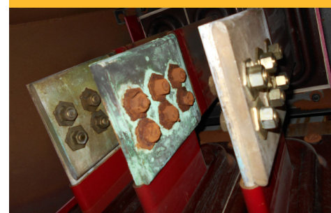
PROBLEM: DIRT/LACK OF SILVER PLATING
