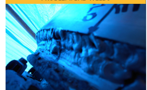
PROBLEM: BAD WELDS
