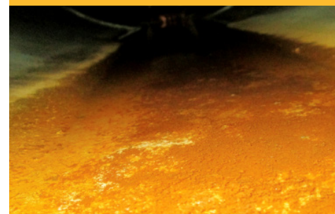
PROBLEM: WATER INTRUSION
